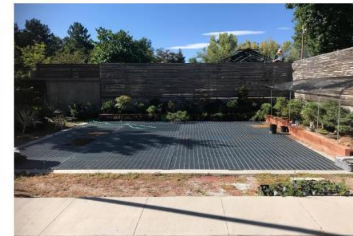
Photograph SF-2. Underground sand filter at Denver Botanic Gardens has a grated top, which enables inspection and maintenance.
