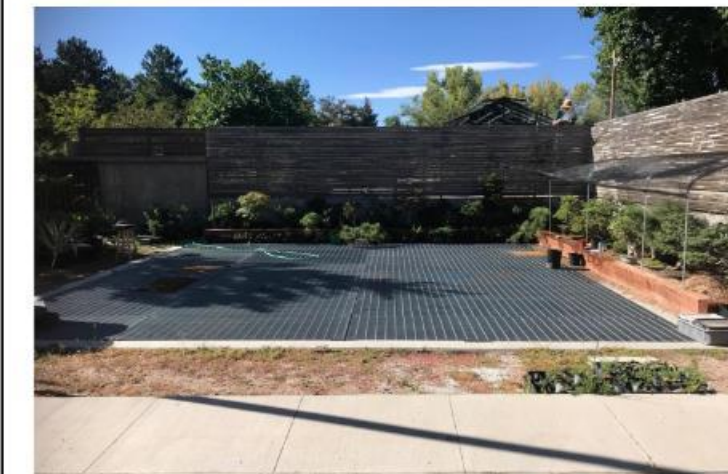
Photograph SF-2. Underground sand filter at Denver Botanic Gardens has a grated top, which enables inspection and maintenance.
