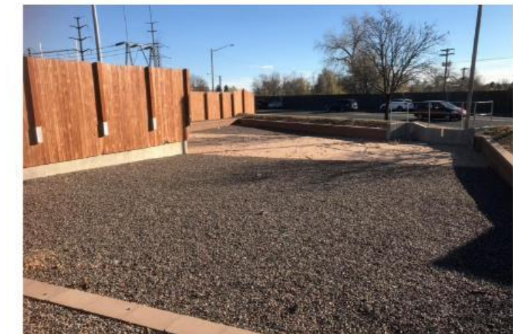
Photograph SF-3. Sand filter with incorporation of minor event flood attenuation provides water quality and detention for a substation.
