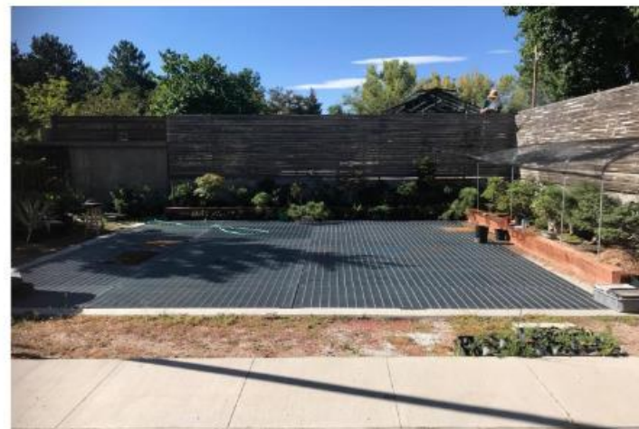
Photograph SF-2. Underground sand filter at Denver Botanic Gardens has a grated top, which enables inspection and maintenance.
