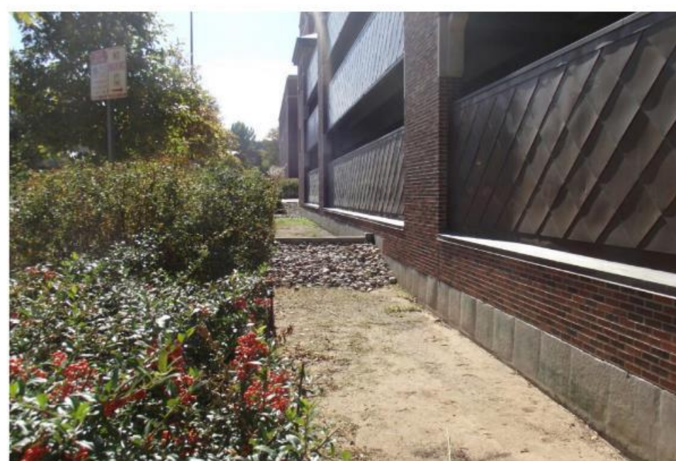
Photograph SF-1. This sand filter, constructed on two sides of a parking garage, is accessible for maintenance, yet screened from public view by a landscape buffer.
