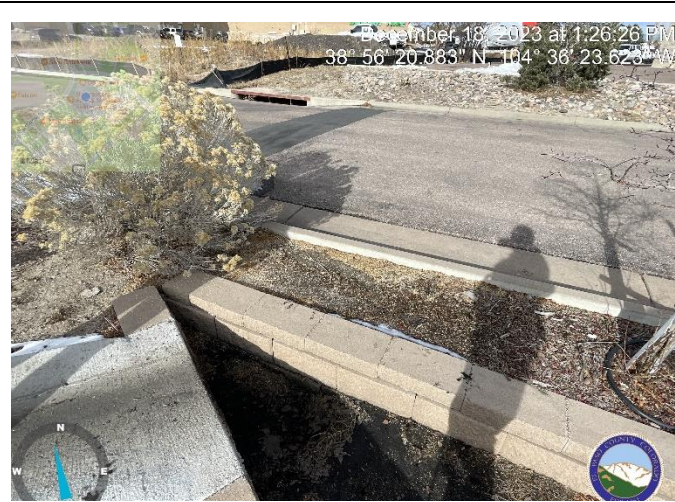
Photo 1: Verify on as-builts, the missing 3' overflow curb cut.
