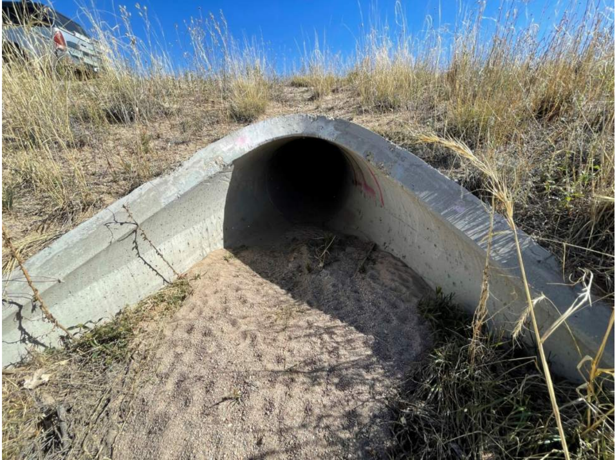
Figure 5: Outlets of pipes into the pond have built up with sediment over time and there is no energy dissipation installed. Type VL rip-rap is to be installed.
