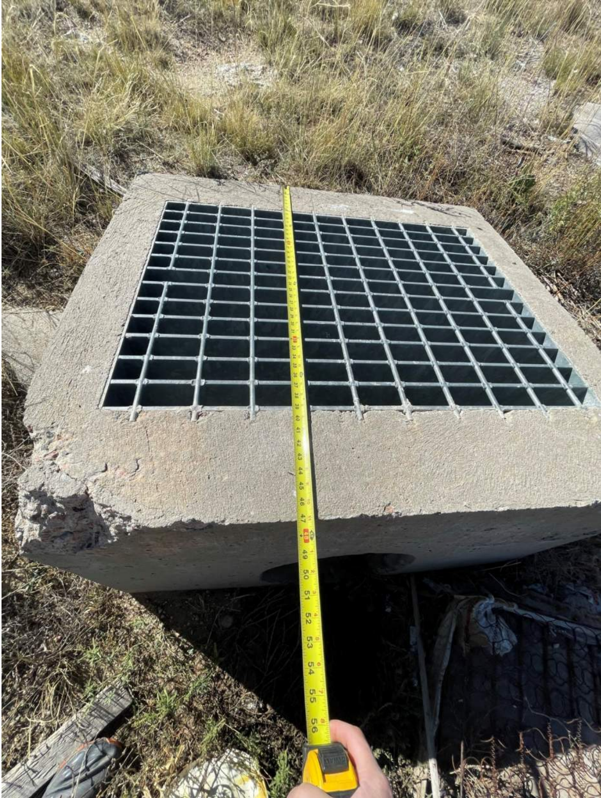
Figure 3: Measurements were taken to ensure that the outlet structure was constructed according to the Construction Drawings. A trash rack was installed per the detail.
