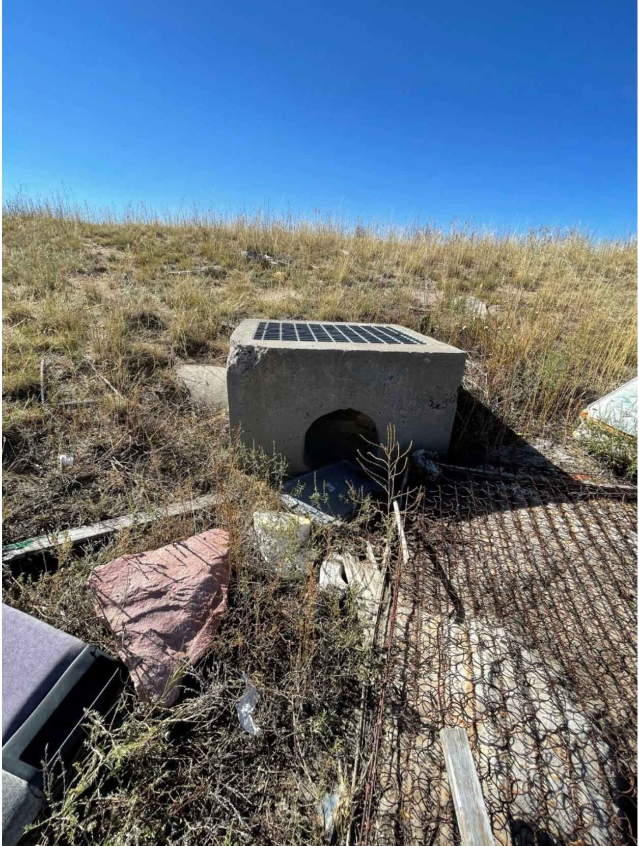
Figure 2: Existing Outlet Structure is in sufficient condition. Dimensions match the Construction Drawings.
