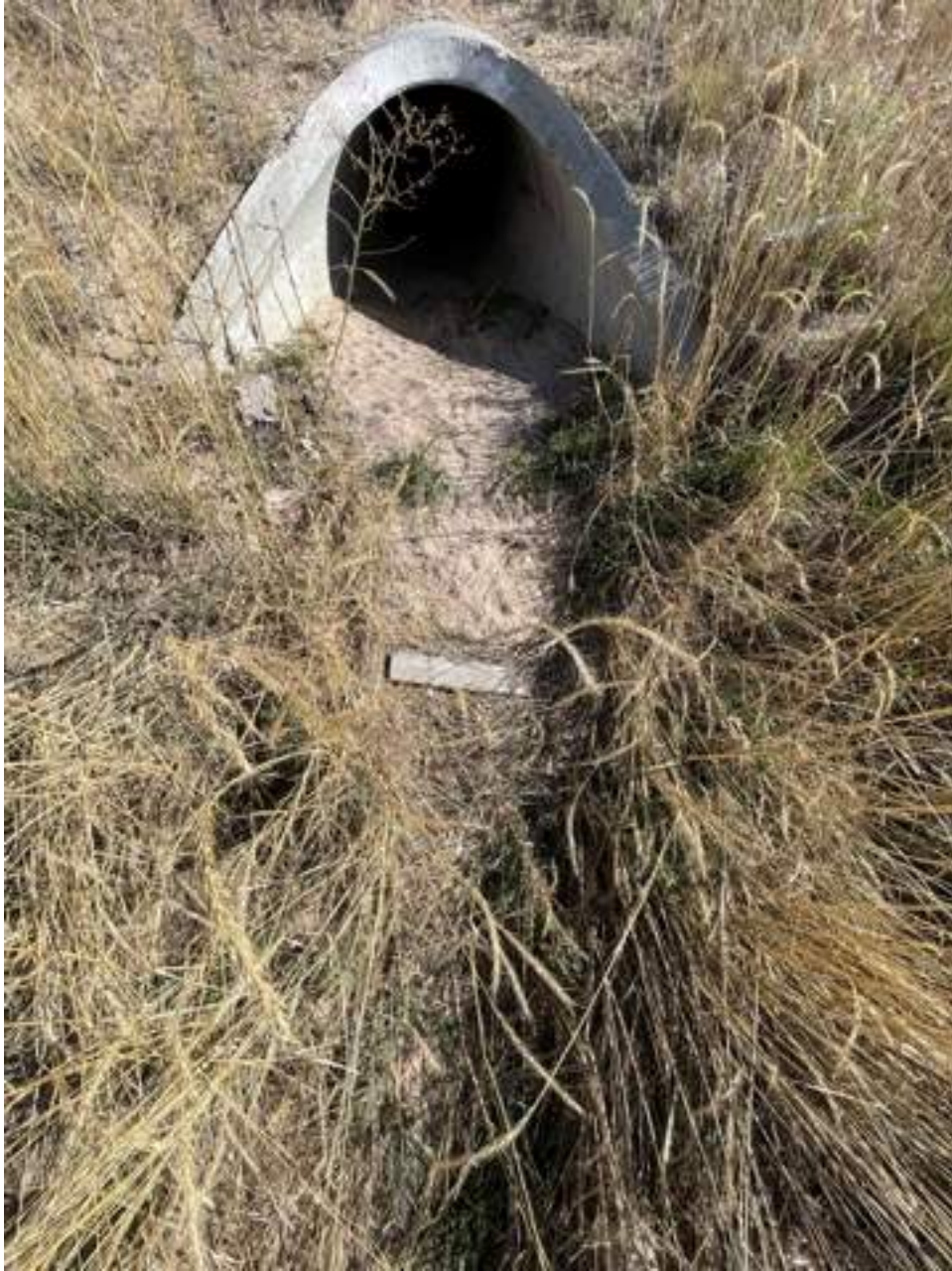
Figure 4: Outlets of pipes into the pond have built up with sediment over time and there is no energy dissipation installed. Type VL rip-rap is to be installed.
