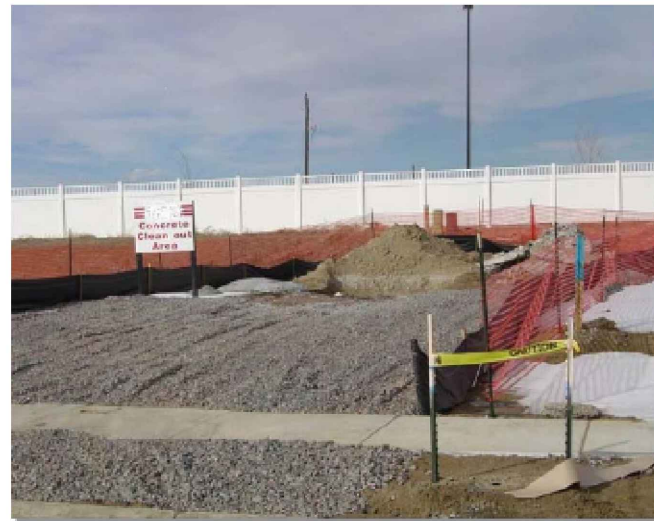
Photograph CWA-1. Example of concrete washout area. Note gravel tracking pad for access and sign.
