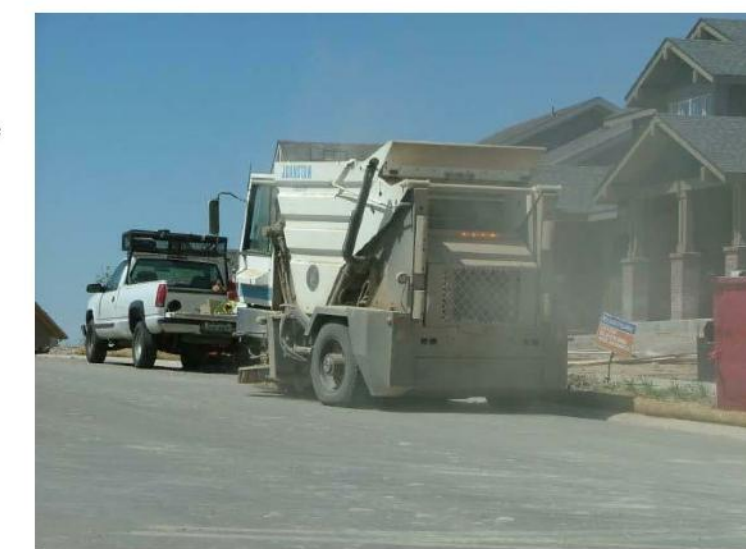
Photograph SS-1. A street sweeper removes sediment and potential pollutants along the curb line at a construction site. Photo courtesy of Tom Gore.
