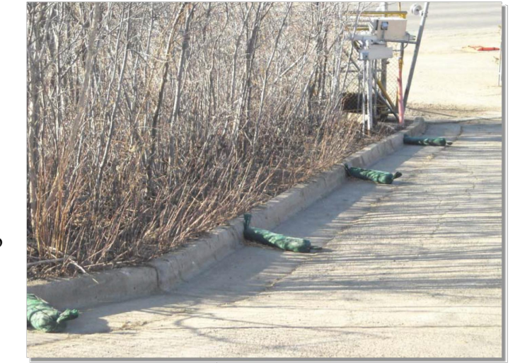
Photograph RS-1. Rock socks placed at regular intervals in a curb line can help reduce sediment loading to storm sewer inlets. Rock socks can also be used as perimeter controls.
