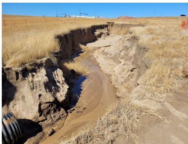
Erosion in Drainage Channel
