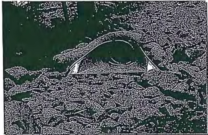
Photograph TOP-1. Riprap outlet protection.
