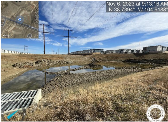
Photo 13: Pond C2.2: Remove debris and sediment from trickle channel, outlet structure, micropool, and forebay.
