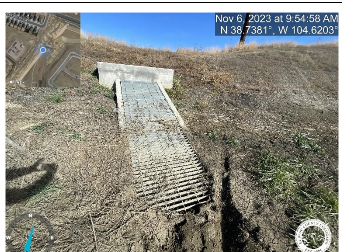
Photo 2: Pond C1: Remove debris and sediment from outfall structure micropool.
