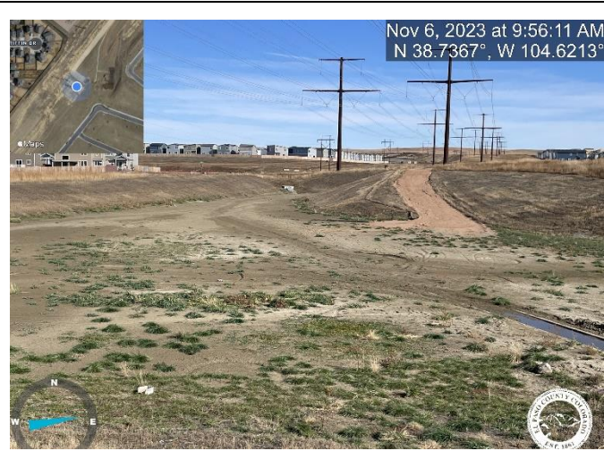
Photo 5: Pond C1: Grade pond bottom to match approved specs and Reinstall maintenance access road per plans. Plans call for 12" deep road base.
