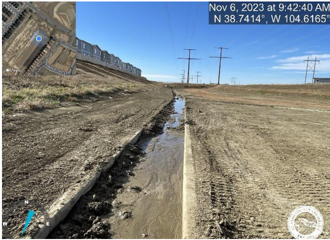
Photo 21: Pond C3: Remove debris and sediment from forebays, trickle channel and outlet structure micropool.
