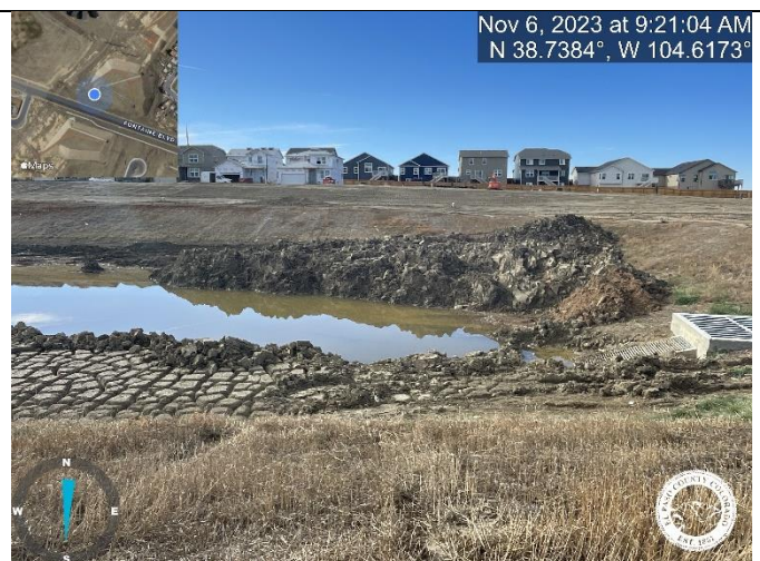
Photo 8: Pond C2.1: Grade pond bottom to match approved specs and Reinstall maintenance access road per plans. Plans call for 12" deep road base.
