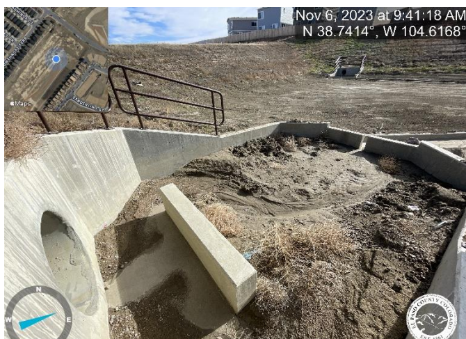
Photo 19: Pond C3: Remove debris and sediment from forebays, trickle channel and outlet structure micropool.
