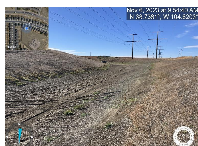
Photo 3: Pond C1: Remove debris and sediment from trickle channel, outlet structure, micropool, and forebay.
