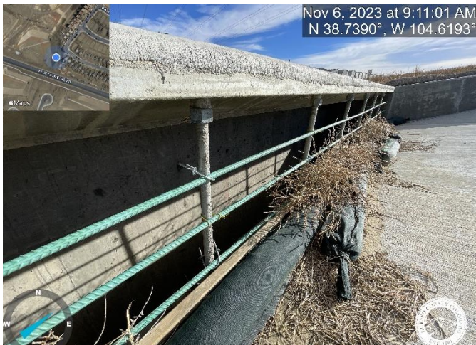
Photo 15: Pond C2.3: Install spillway inlet bars per detail. Approved detail calls for #4 epoxy rebar welded to existing vertical rods. The current installation of U-bolts and tied wire is not adequate.
