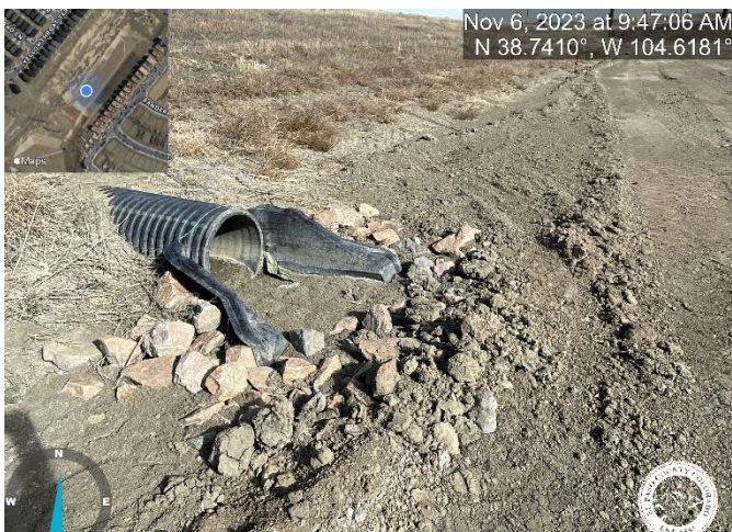
Photo 23: Pond C3: Reestablish the 15'x10' riprap pad at the outfall of the 18" HDPE FES. Reference sheet C9.8 of the Construction Plans.
