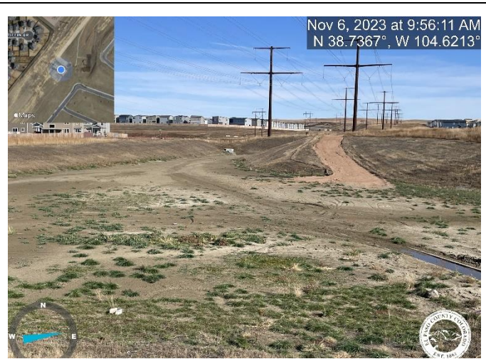
Photo 4: Pond C1: Repair crack in concrete where forebay 1 meets the trickle channel. Item will be checked once pond is cleaned.
