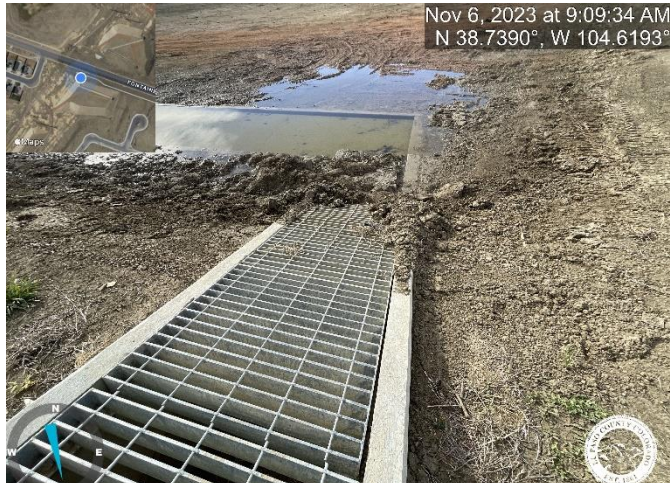
Photo 17: Pond C2.3: Remove debris and sediment from outfall structure micropool.
