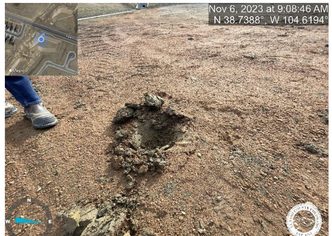
Photo 16: Pond C2.3: Reinstall maintenance access road per plans. Plans call for 12" deep road base. Current road base does not meet minimum specs.
