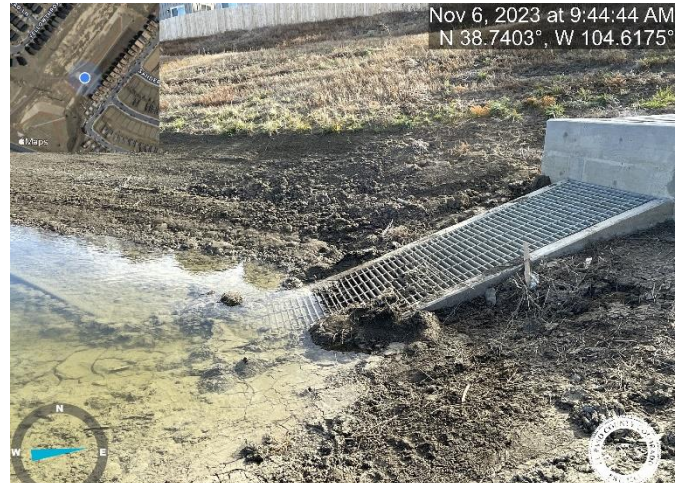
Photo 22: Pond C3: Remove debris and sediment from forebays, trickle channel and outlet structure micropool.
