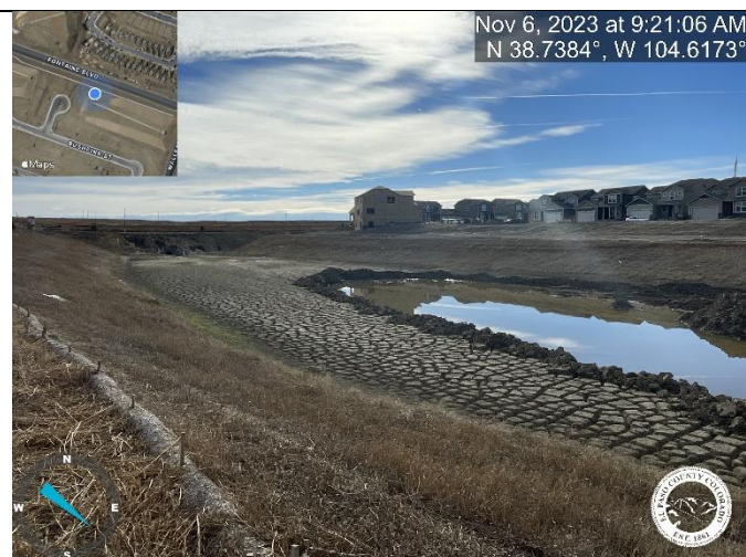
Photo 7: Pond C2.1: Remove debris and sediment from trickle channel, outlet structure, micropool, and forebay.
