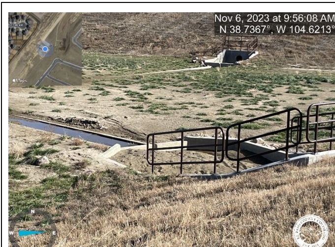
Photo 1: Pond C1: Repair cracking at south forebay pipe entrance. Item will be checked once pond is cleaned.
