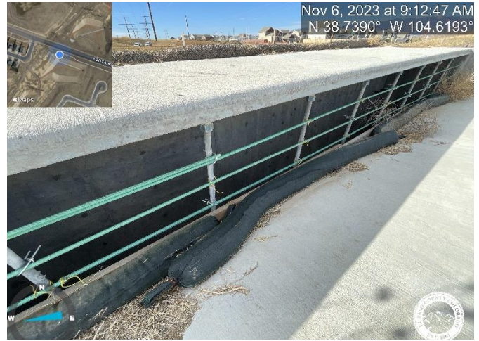
Photo 14: Pond C2.2: Install spillway inlet bars per detail. Approved detail calls for #4 epoxy rebar welded to existing vertical rods. The current installation of U-bolts and tied wire is not adequate.
