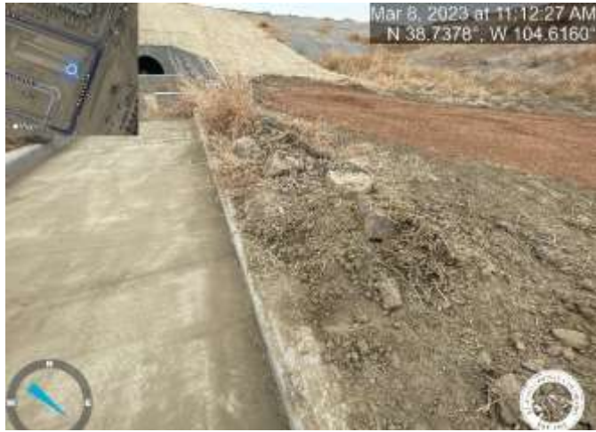
Photo 9: Pond C2.1: Remove sediment to match the top of trickle channel curb with a 3% slope towards trickle channel for positive drainage.
