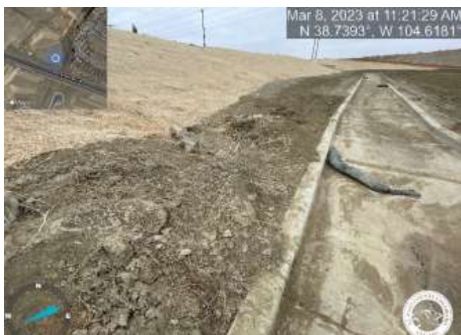
Photo 12: Pond C2.2: Remove sediment to match the top of trickle channel curb with a 3% slope towards trickle channel for positive drainage.
