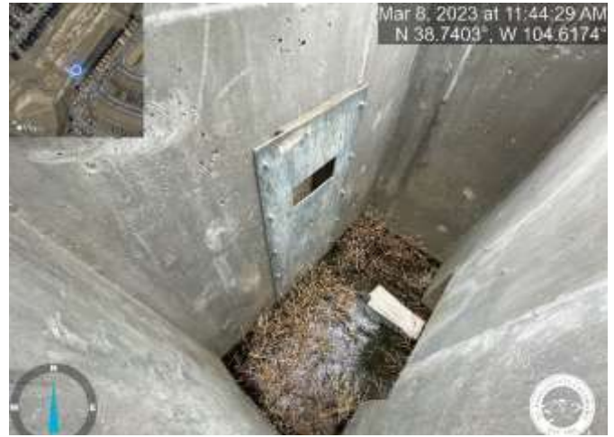
Photo 22: Pond C3: Orifice plate was not properly installed. Invert of the bottom most hole should be at the same elevation as the invert of the outlet pipe.
