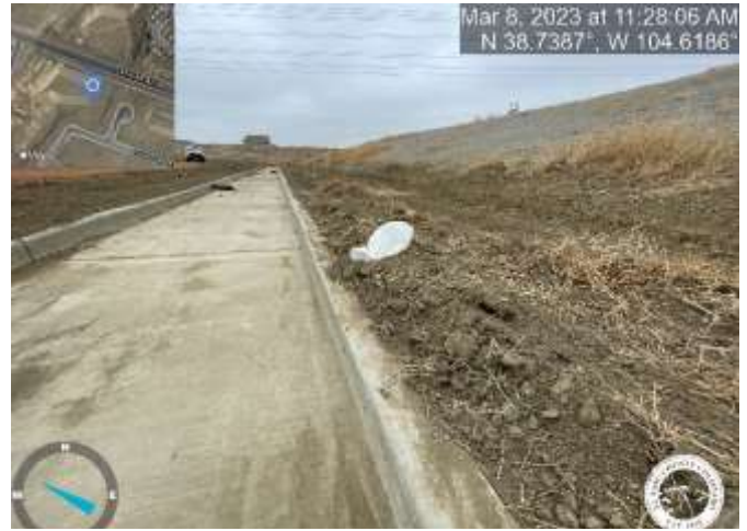
Photo 18: Pond C2.3: Remove sediment to match the top of trickle channel curb with a 3% slope towards trickle channel for positive drainage.
