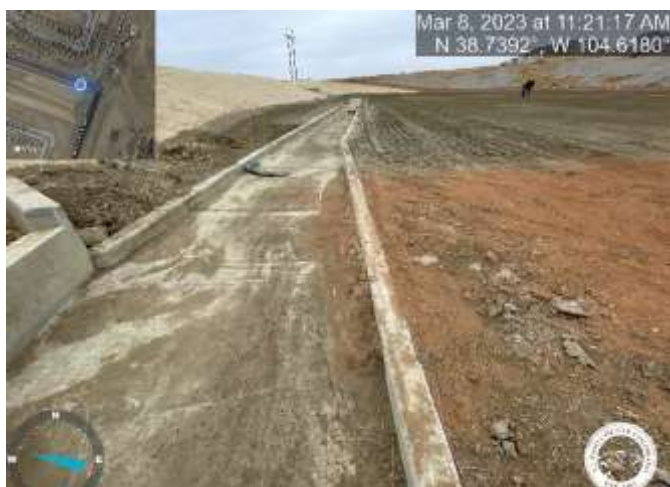
Photo 11: Pond C2.2: Remove excess sediment and road base from the trickle channel.
