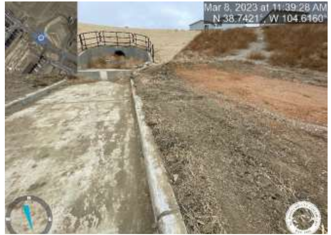
Photo 26: Pond C4: Remove excess sediment from trickle channel and old/damaged straw wattles.
