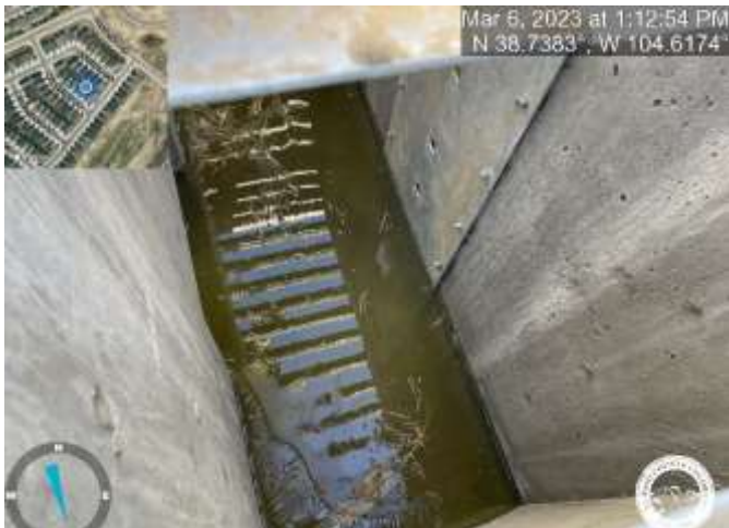
Photo 7: Pond C2.1: Orifice plate was not properly installed. Invert of the bottom most hole should be at the same elevation as the invert of the outlet pipe.
