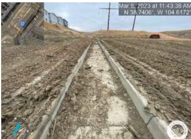
Photo 19: Pond C3: Remove excess sediment from trickle and match grade the top of trickle channel curb with a 3% slope towards trickle channel for positive drainage.
