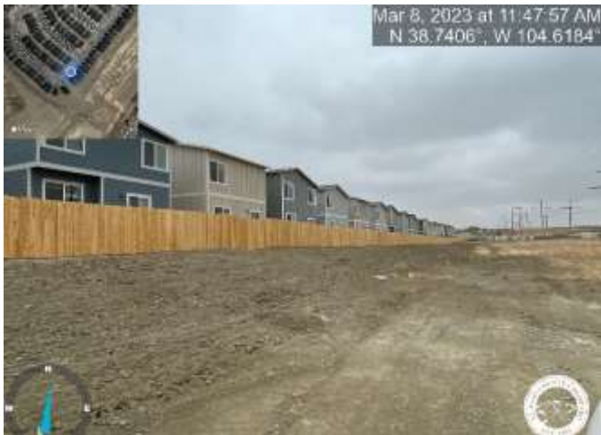
Photo 31: East perimeter of Area 'B': Failure to implement permanent seeding.
