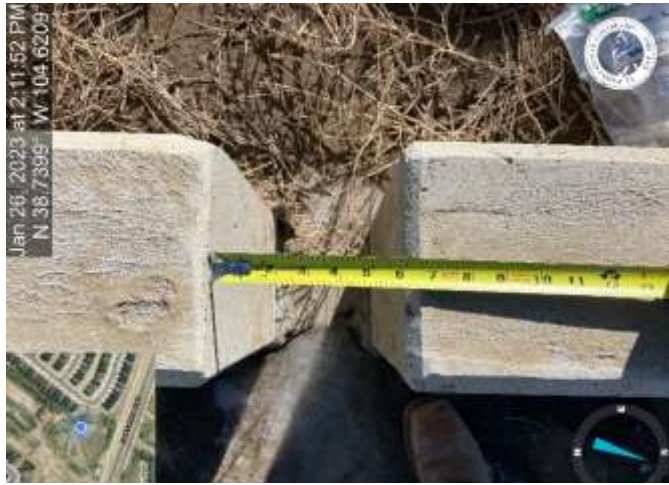
Photo 10: Pond C2.2: Notch on Forebay 'A' should be cut to 8". Reference sheet C9.6 on the CD's.
