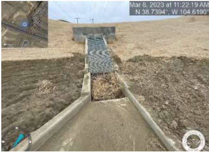
Photo 13: Pond C2.2: Match grade the top of trickle channel curb with a 3% slope towards trickle channel for positive drainage.
