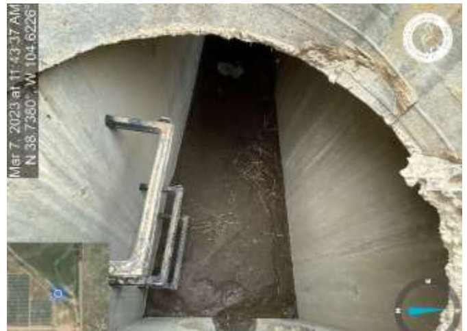
Photo 32: Remove sediment and debris from inlets throughout site. Inlets are marked with a green dot on the lid (approximately 23 inlets).
