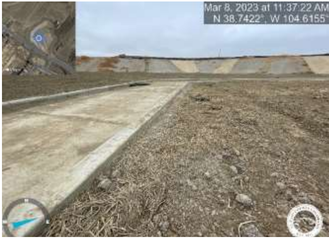
Photo 25: Pond C4: Raise pond bottom to top of trickle channel curb with a 3% slope towards trickle channel for positive drainage.
