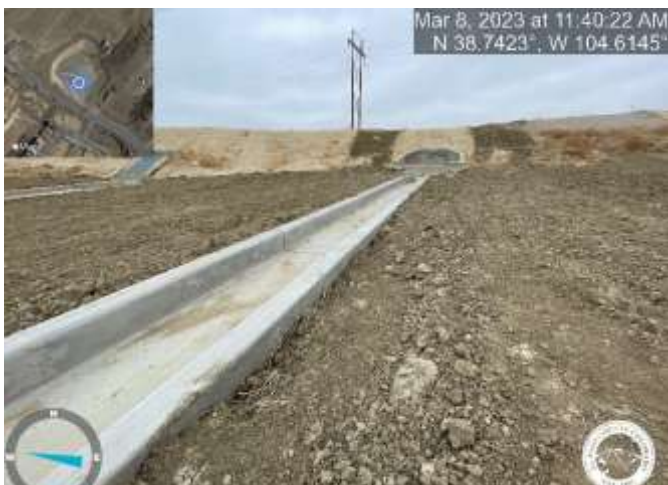
Photo 27: Pond C4: Raise pond bottom to top of trickle channel curb with a 3% slope towards trickle channel for positive drainage.
