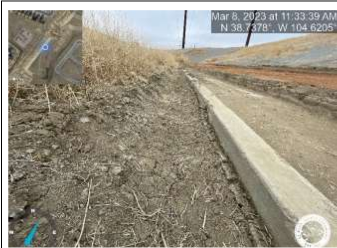
Photo 3: Pond C1: Raise pond bottom to top of trickle channel curb with a 3% slope towards trickle channel for positive drainage.
