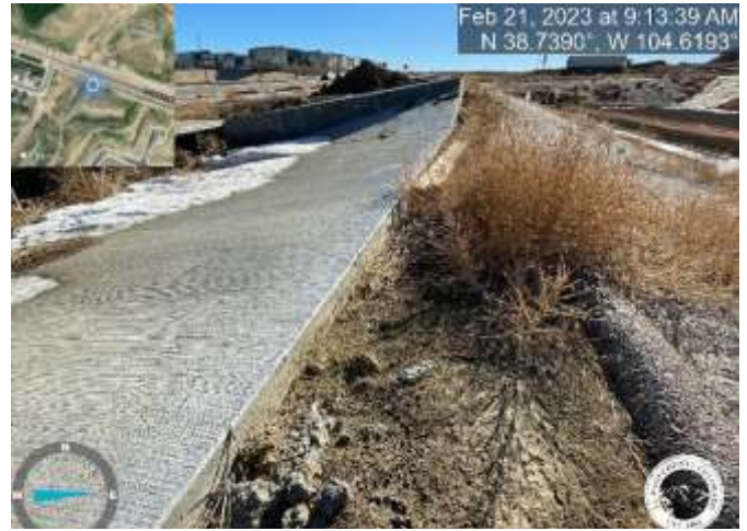
Photo 30: Emergency overflow form pond C2.3: Raise grade to be flush with overflow structure.
