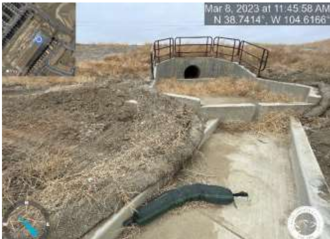
Photo 23: Pond C3: Remove old/damaged straw wattles from forebay.
