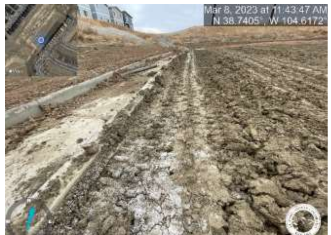
Photo 20: Pond C3: Remove excess sediment from trickle and match grade the top of trickle channel curb with a 3% slope towards trickle channel for positive drainage.
