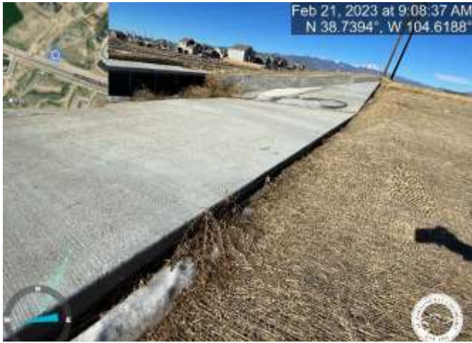
Photo 29: Emergency overflow form pond C2.2: Raise grade to be flush with overflow structure.
