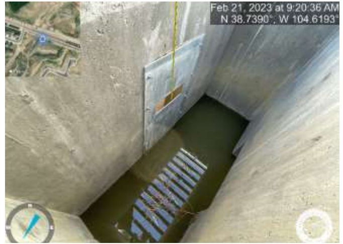
Photo 14: Pond C2.3: Orifice plate was not properly installed. Invert of the bottom most hole should be at the same elevation as the invert of the outlet pipe.
