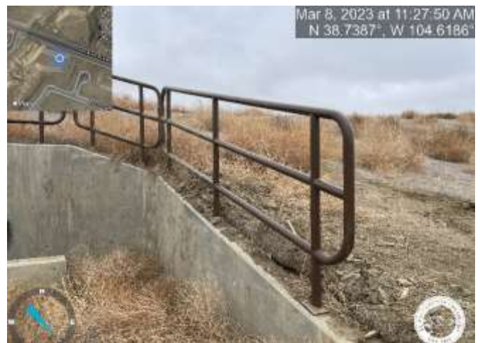
Photo 16: Pond C2.3: Remove excess sediment and damaged straw wattles around forebay.
