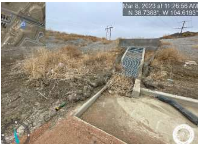
Photo 15: Pond C2.3: Remove excess sediment and damaged straw wattles around outlet structure.
