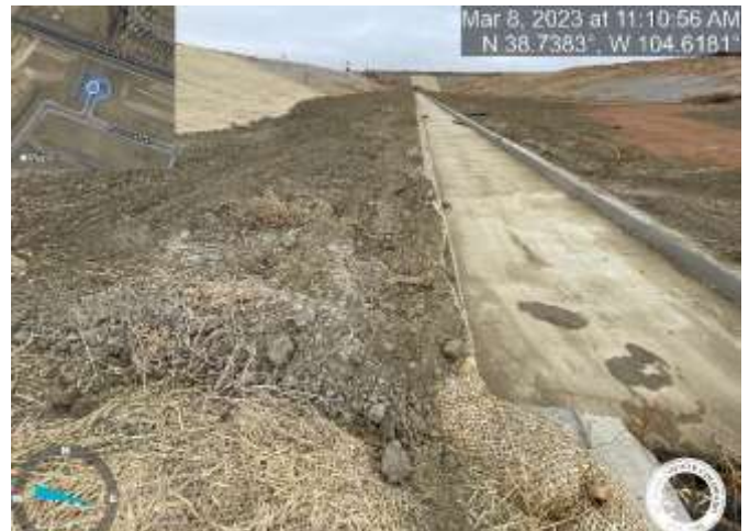
Photo 8: Pond C2.1: Remove sediment to match the top of trickle channel curb with a 3% slope towards trickle channel for positive drainage.
