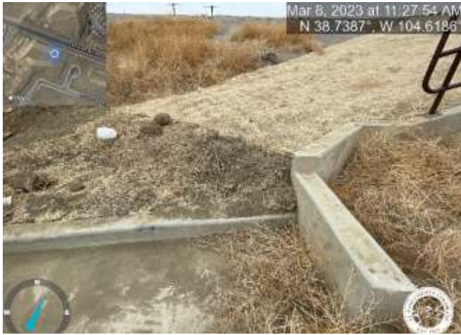
Photo 17: Pond C2.3: Remove sediment to match the top of trickle channel curb with a 3% slope towards trickle channel for positive drainage.
