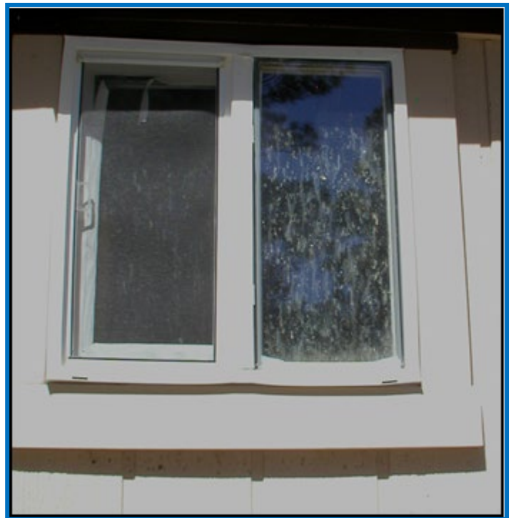
The vinyl window frame on this home melted and warped in the Black Forest Fire, but not enough to allow firebrands inside the home. Metal framed windows resist warping.
