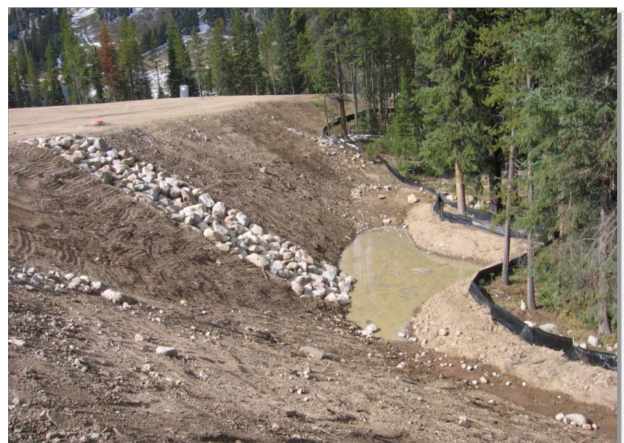
Photograph SB-1. Sediment basin at the toe of a slope. Photo courtesy of W.W.E.
