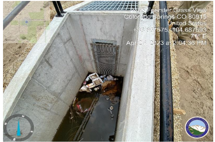
Photo 10: Well screen not installed per specification. (Pond B Page 29)
