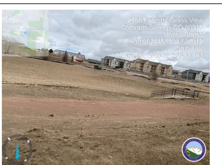
Photo 16: Maintenance road not installed per specification (Pond B Page 31)
