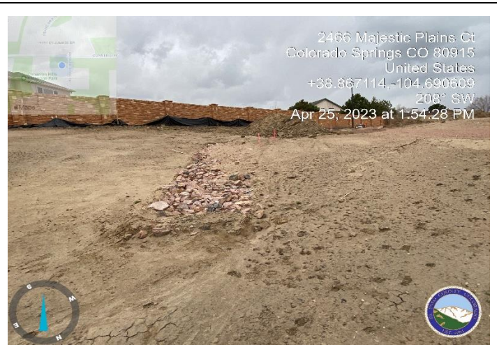
Photo 8: Riprap rundown not built per plans (Page 27 of CDs)
