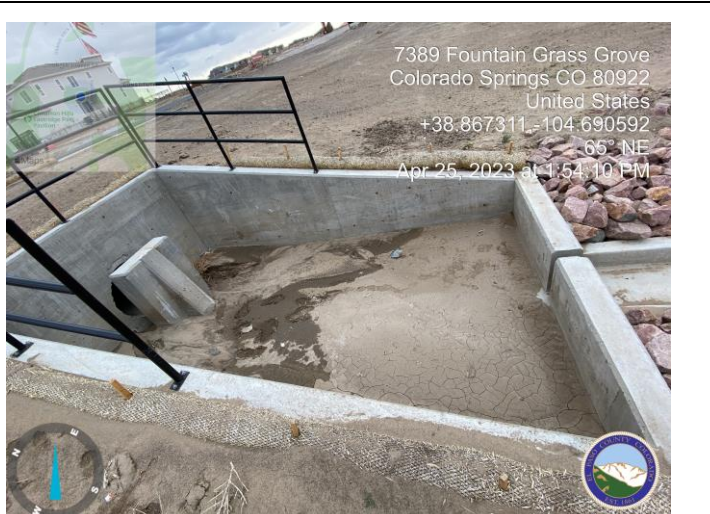
Photo 14: Ponds A & B. Clean out sediment and debris from outlet structure and trickle channels.
