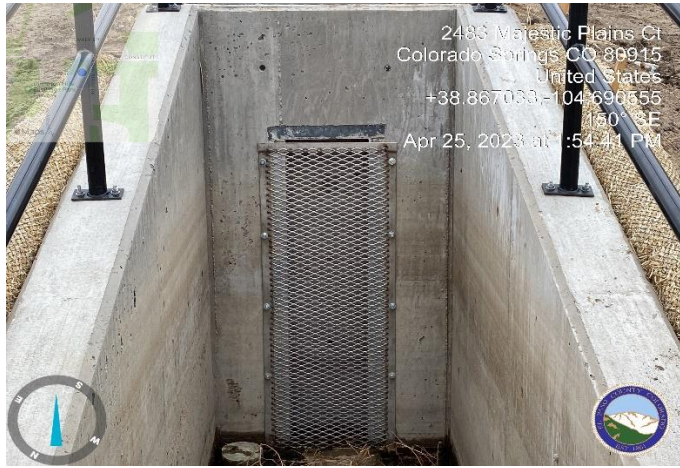
Photo 9: Well screen not installed per specification. (Pond A page 25)
