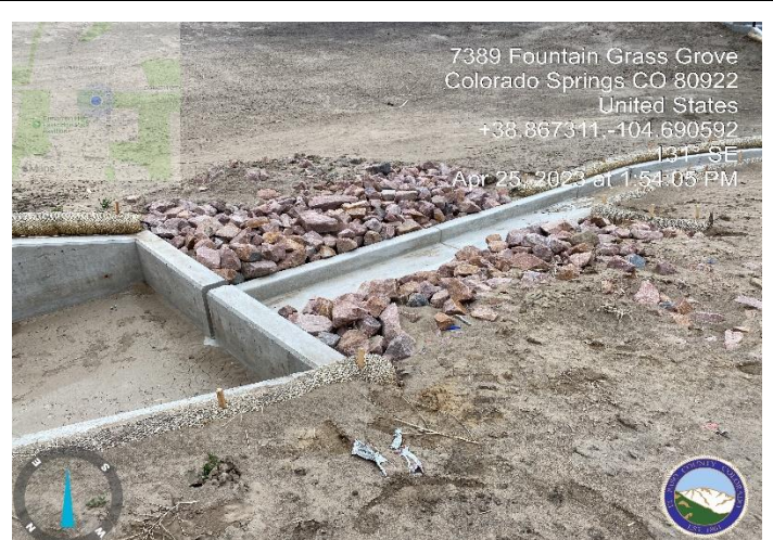
Photo 6: Pond A Soil Rip Rap not installed per specification. (Page 27 of CD'S) Soiled Rip rap must be flush with top of trickle channel and premixed before installation.
