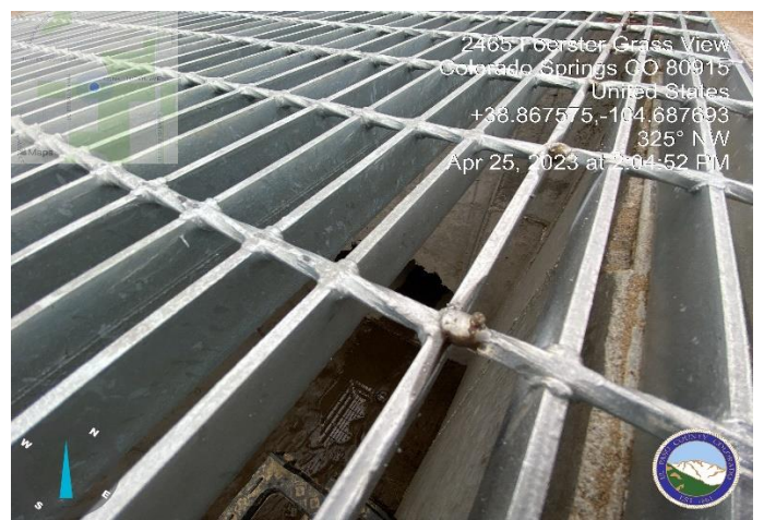
Photo 12: Restrictor plates missing. (Pond B Page 30)
