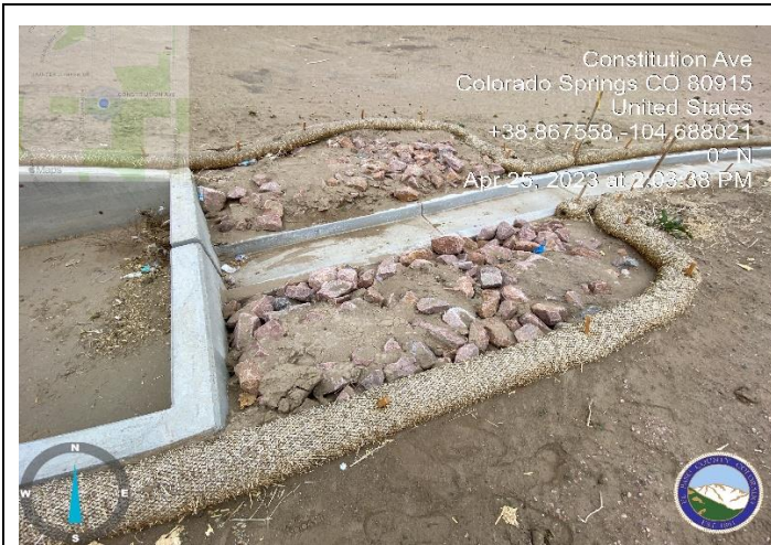
Photo 7: Pond B soil riprap not installed per plans. Soil riprap must be flush with top of trickle channel and pre-mixed before installed
