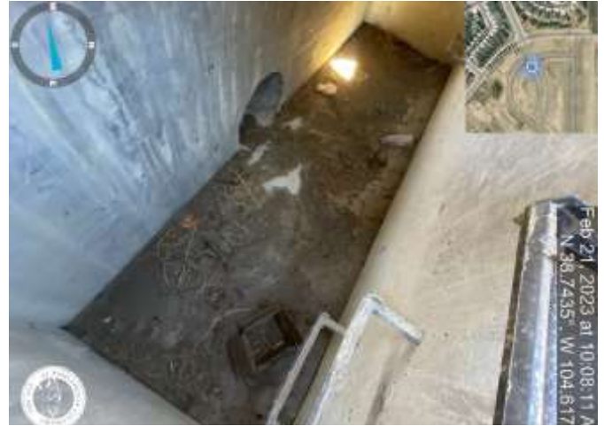
Photo 2: Inlet DP38c: Remove sediment and debris from inlet (inlet is marked with a green dot on the lid).
