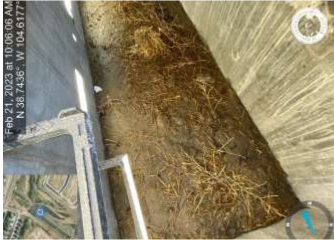
Photo 1: Inlet DP38a: Remove sediment and debris from inlet (inlet is marked with a green dot on the lid).
