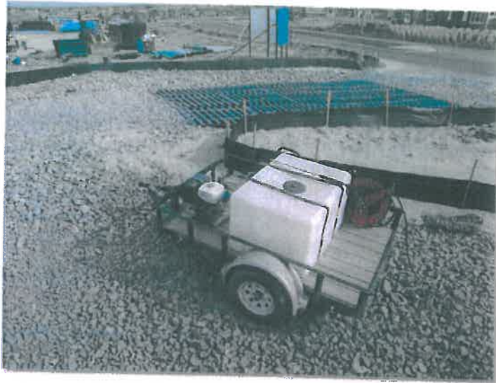
Photograph VTC-2. A vehicle tracking control pad with wheel wash facility. Photo courtesy of Tom Gore.
