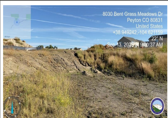
Photo 6: North Pond embankments eroding. Regrade and stabilize.
