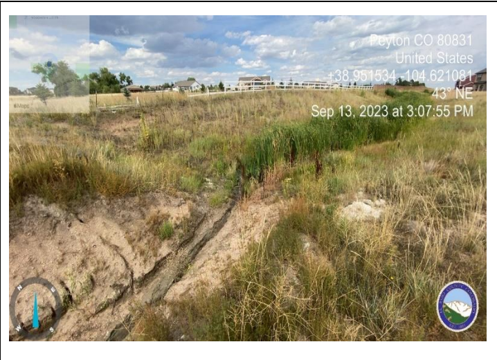
Photo 10: Swale A has standing water at point near channel. Cat tails present. Sediment eroding into channel. Regrade to promote positive drainage and stabilize.
