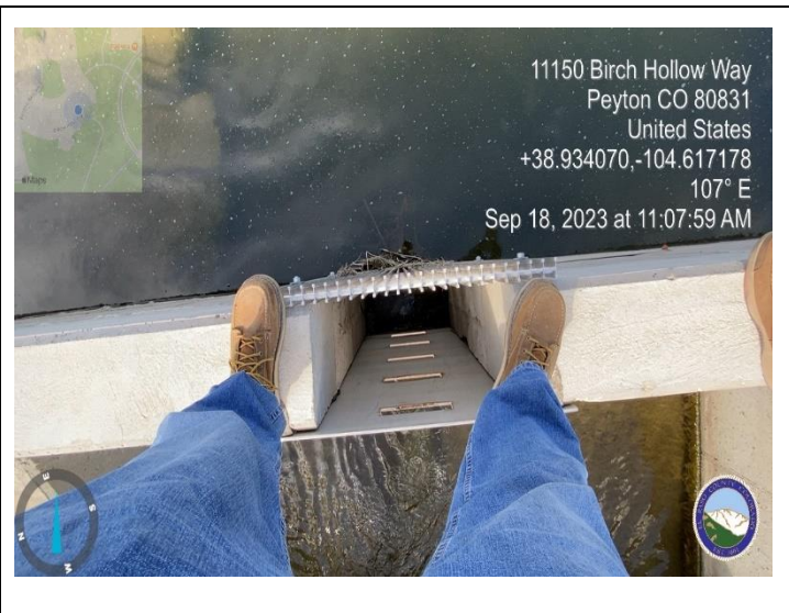
Photo 12: Pond WU - Install plate over cross member to prevent debris clogging outlet structure.
