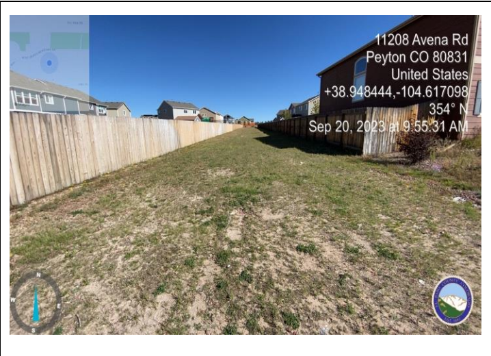
Photo 14: Swale G not Installed per plan
