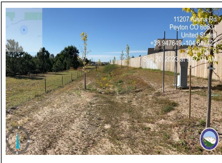
Photo 15: Swale H not installed per plan
