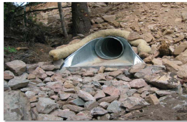
Photograph TOP-1. Riprap outlet protection.
