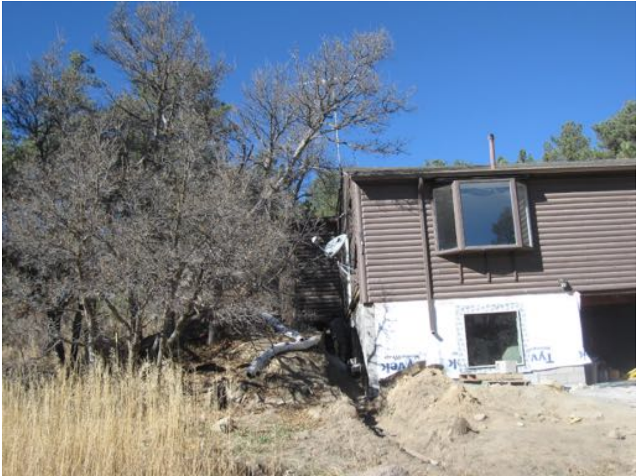
Photo 5. Oak limbs overhanging an existing structure and opportunity to prune away from the upper combustible wood siding.
