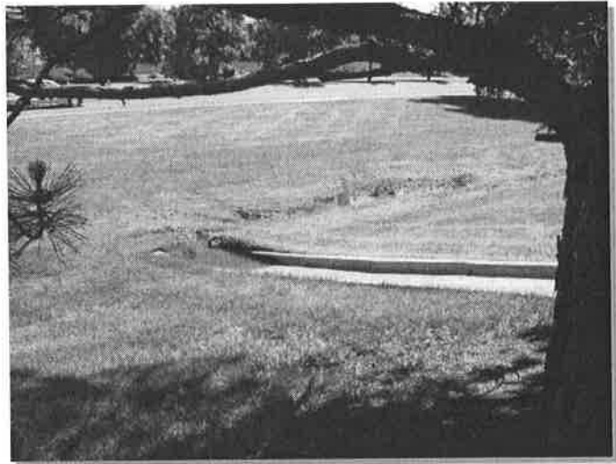
Photograph 6-2. A lack of sediment removal in this grass swale has resulted in a grade change due to growth over the deposition and ponding upstream.
