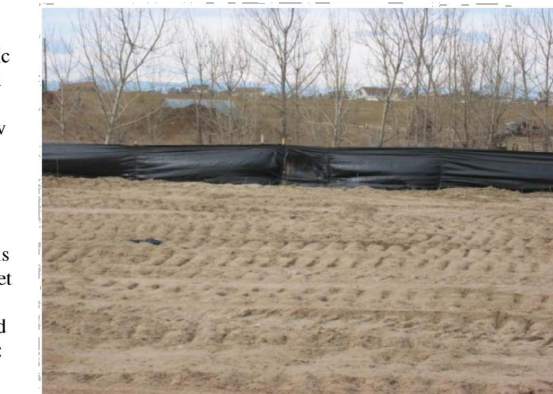
Photograph SF-1. Silt fence creates a sediment barrier, forcing sheet flow runoff to evaporate or infiltrate.
