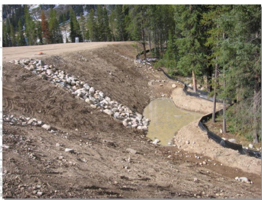
Photograph SB-1. Sediment basin at the toe of a slope. Photo courtesy of WWT.
