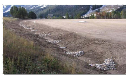
Photograph CD-1. Rock check dam in a roadside ditch. Photo courtesy of WVE.
