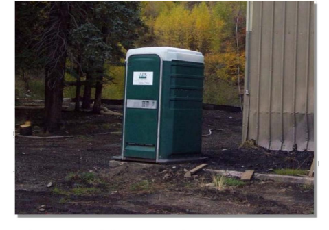
Photograph GH-3. Locate portable toilet facilities on level surfaces away from waterways and storm drains. Photo courtesy of WWT.
