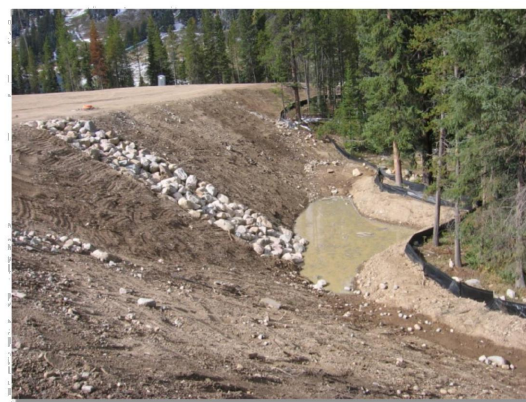
Photograph SB-1. Sediment basin at the toe of a slope. Photo courtesy of WWT.
