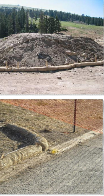
Photographs SCL-1 and SCL-2. Sediment control logs used as 1) a perimeter control around a stockpile and, 2) as a "J-hook" perimeter control at the corner of a construction site.
