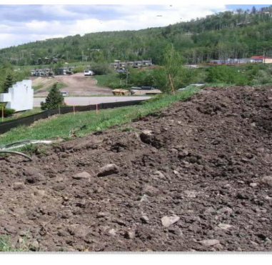
Photograph SP-1. A topsoil stockpile that has been partially revegetated and is protected by silt fence perimeter control.
