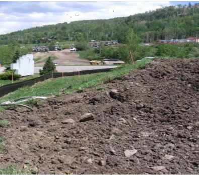
Photograph SP-1. A topsoil stockpile that has been partially revegetated and is protected by silt fence perimeter control.
