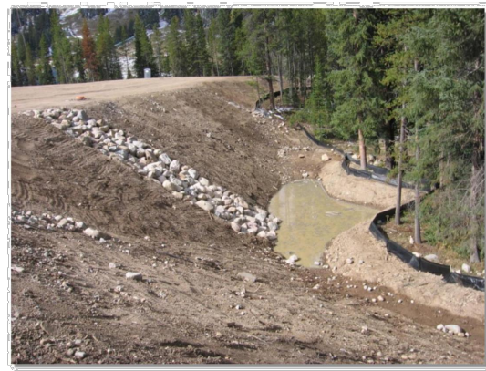
Photograph SB-1. Sediment basin at the toe of a slope. Photo courtesy of WWH.
