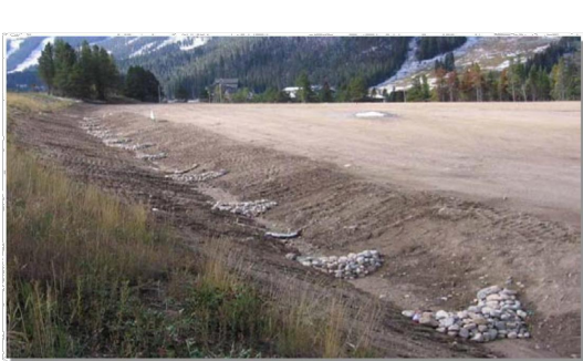
Photograph CD-4: Rock check dam in a washable ditch. Photo courtesy of WWE.
