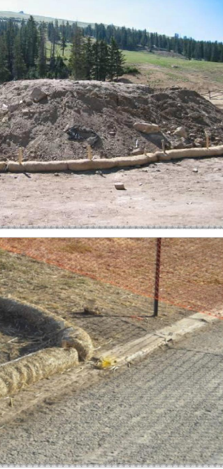
Photographs SCL-1 and SCL-2. Sediment control logs used as 1) a perimeter control around a stockpile and, 2) as a "J-hook" perimeter control at the corner of a construction site.
