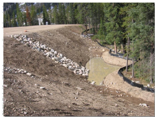
Photograph SB-1. Sediment basin at the toe of a slope. Photo courtesy of UDFCD.
