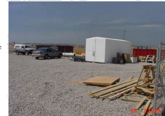
Photograph SSA-1. Example of a staging area with a gravel surface to prevent mud tracking and reduce runoff. Photo courtesy of Douglas County.
