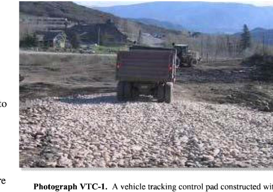
Photograph VTC-1. A vehicle tracking control pad constructed with properly sized rock reduces off-site sediment tracking.
