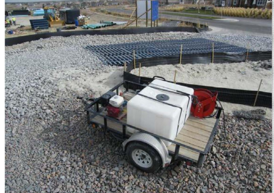
Photograph VTC-2. A vehicle tracking control pad with wheel wash facility. Photo courtesy of Tom Gore.
