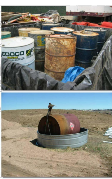
Photographs GH-1 and GH-2. Proper materials staging and secondary containment for fuel tanks are important good housekeeping practices. Photos courtesy of CDOT and City of Aurora.
