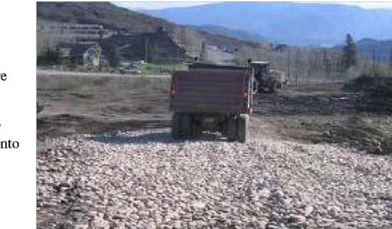
Photograph VTC-1. A vehicle tracking control pad constructed with properly sized rock reduces off-site sediment tracking.
