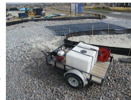
Photograph VTC-2. A vehicle tracking control pad with wheel wash facility. Photo courtesy of Tom Gies.
