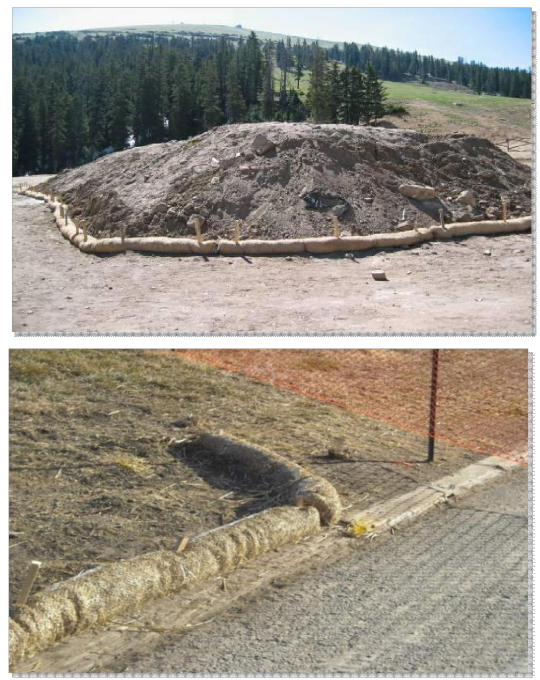
Photographs SCL-1 and SCL-2. Sediment control logs used as 1) a perimeter control around a site, and 2) as a 'J-hook' perimeter control at the corner of a construction site.
