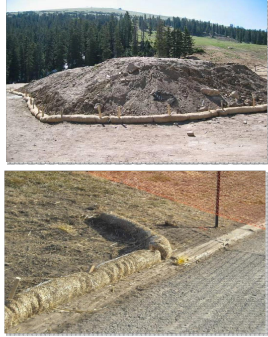
Photographs SCL-1 and SCL-2. Sediment control logs used as 1) a perimeter control around a stockpile and, 2) as a "J-hook" perimeter control at the corner of a construction site.
