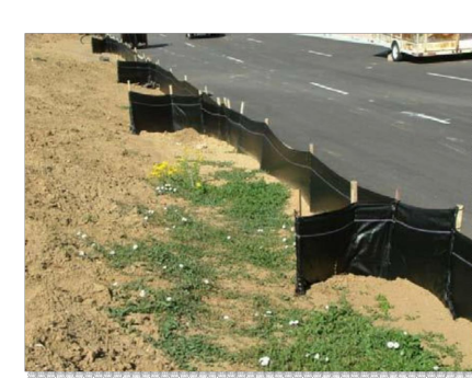
Photograph SF-2. When silt fence is not installed along the contour, a "J-hook" installation may be appropriate to ensure that the BMP does not create concentrated flow parallel to the silt fence. Photo courtesy of Tom Owe.
