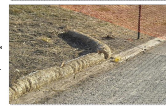
Photographs SCL-1 and SCL-2. Sediment control logs used as 1) a perimeter control around a stockpile and, 2) as a 'J-hook' perimeter control at the corner of a construction site.
