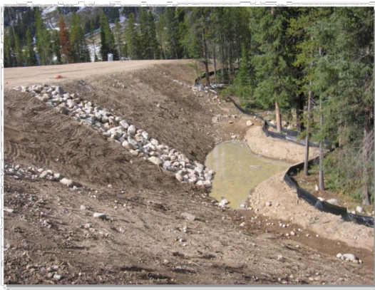
Photograph SB-1. Sediment basin at the toe of a slope. Photo courtesy of WWS.
