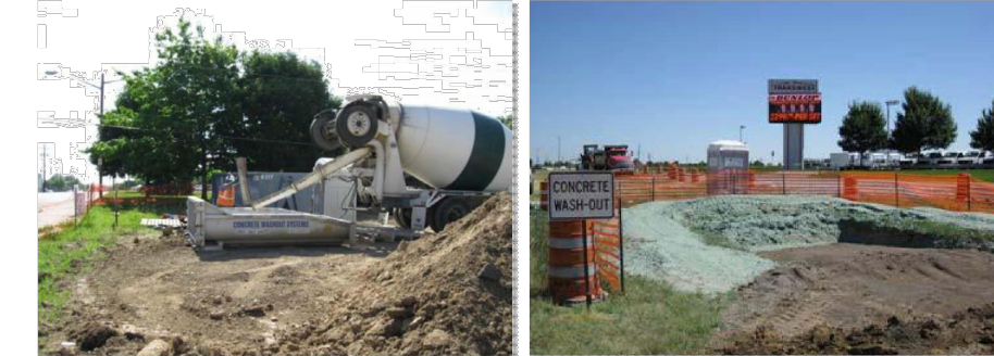
Photograph CWA-2. Prefabricated concrete washout. Photo courtesy of CDOT. Photograph CWA-3. Earthen concrete washout. Photo courtesy of CDOT.
