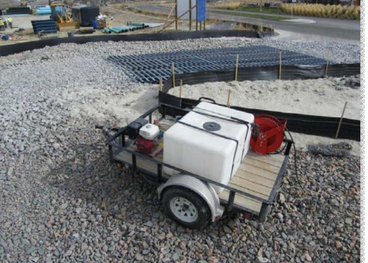
Photograph VTC-2. A vehicle tracking control pad with wheel wash facility. Photo courtesy of Tom Gies.
