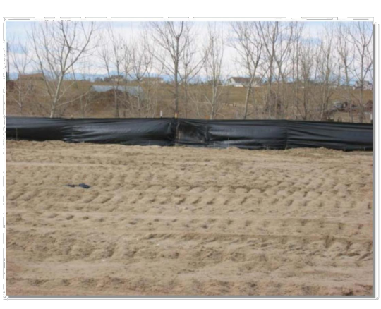
Photograph SF-1. Silt fence creates a sediment barrier, forcing sheet flow runoff to evaporate or infiltrate.
