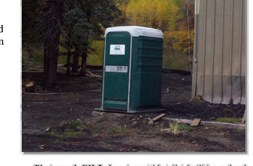
Photograph GH-3. Locate portable toilet facilities on level surfaces away from waterways and storm drains.
