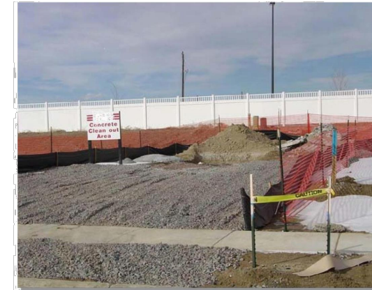
Photograph CWA-1. Example of concrete washout area. Note gravel tracking pad for access and signs.
