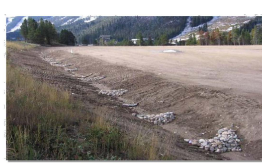
Photograph CD-1. Rock check dam in a roadside ditch. Photo courtesy of WWE.
