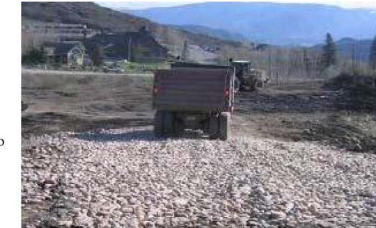
Photograph VTC-1. A vehicle tracking control pad constructed with properly sized rock reduces off-site sediment tracking.
