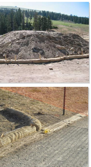
Photographs SCL-1 and SCL-2. Sediment control logs used as 1) a perimeter control around a stockpile and, 2) as a "J-hook" perimeter control at the corner of a construction site.
