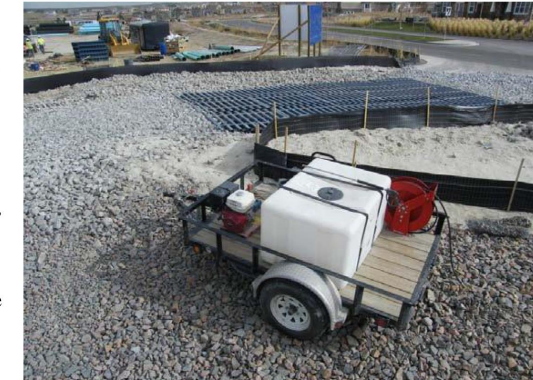
Photograph VTC-2. A vehicle tracking control pad with wheel wash facility. Photo courtesy of Tom Gore.
