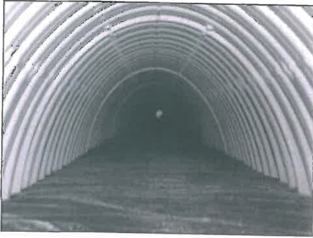
Looking down the Isolator Row from the manhole opening, woven geotextile is shown between the chamber and stone base.
