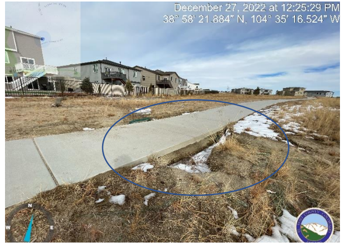
Photo 6: Tract A. Rear of lot 29. Sidewalk is undercut.
