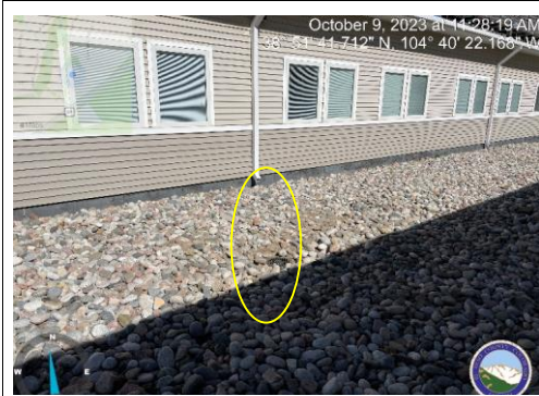
Photo 1: The underdrain system where area drain is present is holding water. Ensure the system is not clogged/broken.
