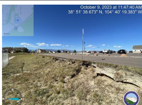
Photo .8: South side of parking/detention pond embankment lot is highly eroded/undercut in multiple locations.
