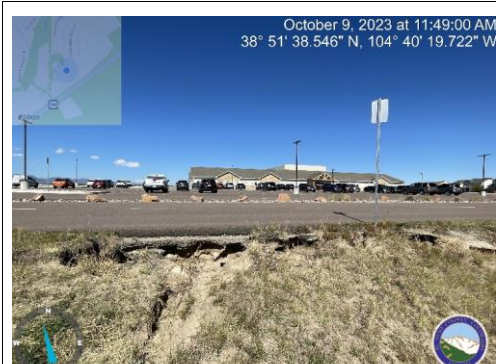
Photo 7: South side of parking/detention pond embankment lot is highly eroded/undercut in multiple locations.
