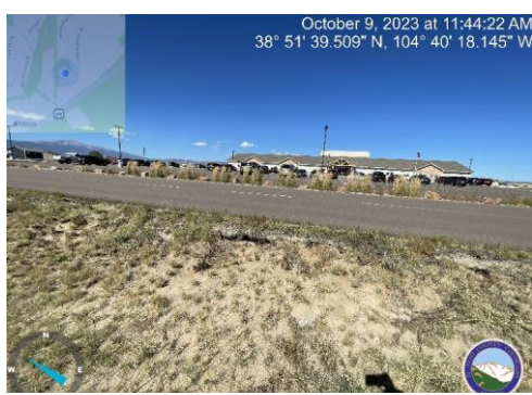
Photo 11: South side of parking/detention pond embankment lot is highly eroded/undercut in multiple locations.
