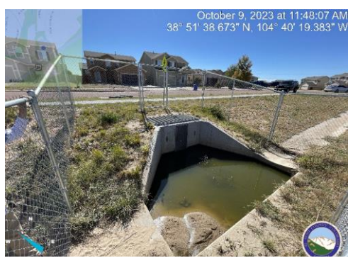
Photo 12: Sediment build up in micro pool of outlet structure needs to be cleaned out.
