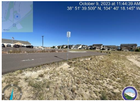
Photo 9: South side of parking/detention pond embankment lot is highly eroded/undercut in multiple locations.
