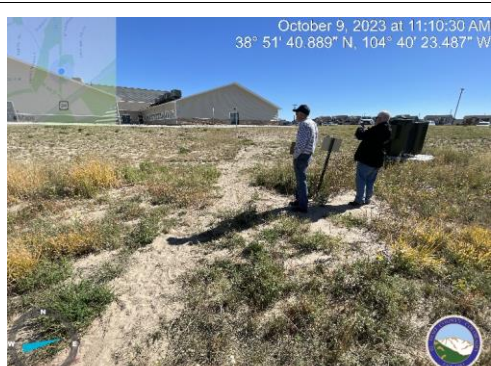
Photo 6: Sparse vegetation, sedimentation, and erosion on Tract A west of the 20' sidewalk location.
