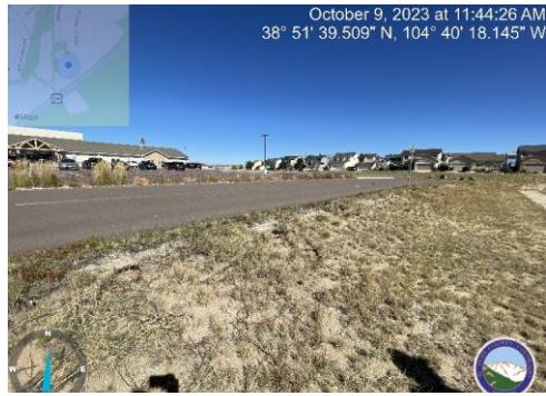
Photo 10: South side of parking/detention pond embankment lot is highly eroded/undercut in multiple locations.
