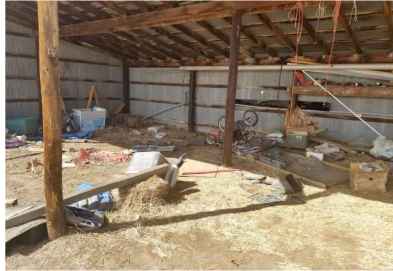
6. Debris and trash observed in open ended barn.
