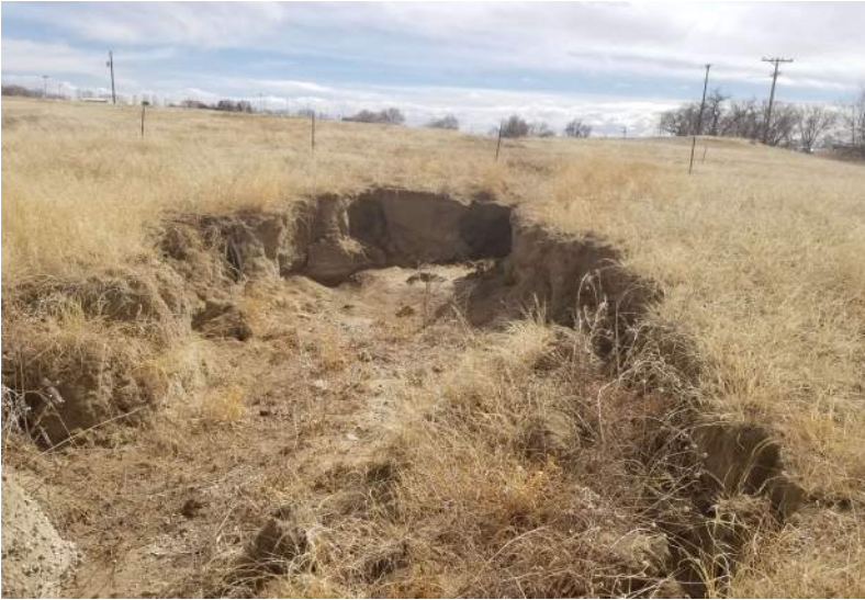
17. Erosion from storm water on west end of site.
