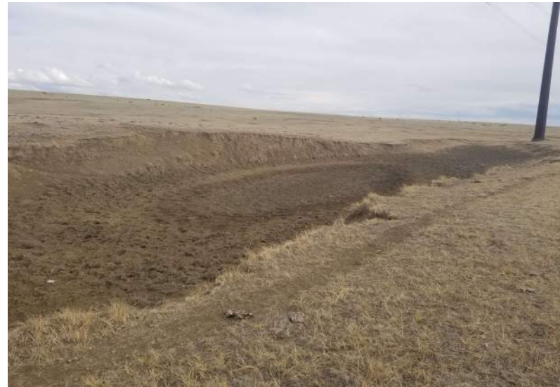
28. Erosion present center of site adjacent to power lines and easement.
