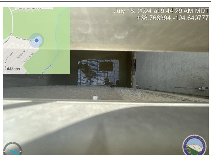
Photo 8: Gasket on orifice plate not sealed. Reinstall.
