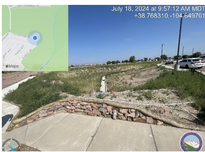
Photo 10: Retaining wall (Approx. 2'H x 22'L) not on approved plans. Include on as built.
