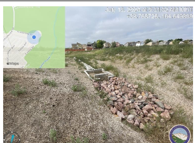
Photo 4: Riprap in front of forebay not on approved plans. Include on as built.
