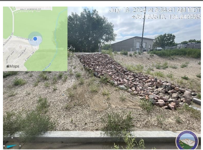
Photo 6: Small blowout on north side of riprap rundown. Eliminate the cause of erosion.
