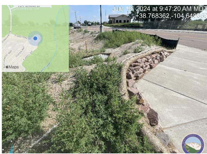
Photo 9: Retaining wall (Approx. 2'H x 22'L) not on approved plans. Include on as built.
