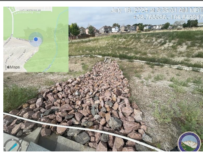
Photo 5: Small blowout on north side of riprap rundown. Eliminate the cause of erosion.
