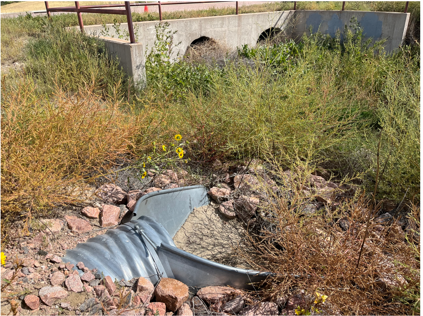
Image taken looking southeast at the existing outfall configuration of the 24" CMP storm sewer line beginning onsite and terminating in Flagstone Channel.
