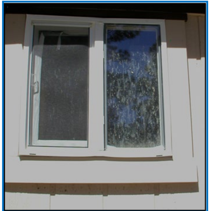
The vinyl window frame on this home melted and warped in the Black Forest Fire, but not enough to allow firebrands inside the home. Metal framed windows resist warping.
