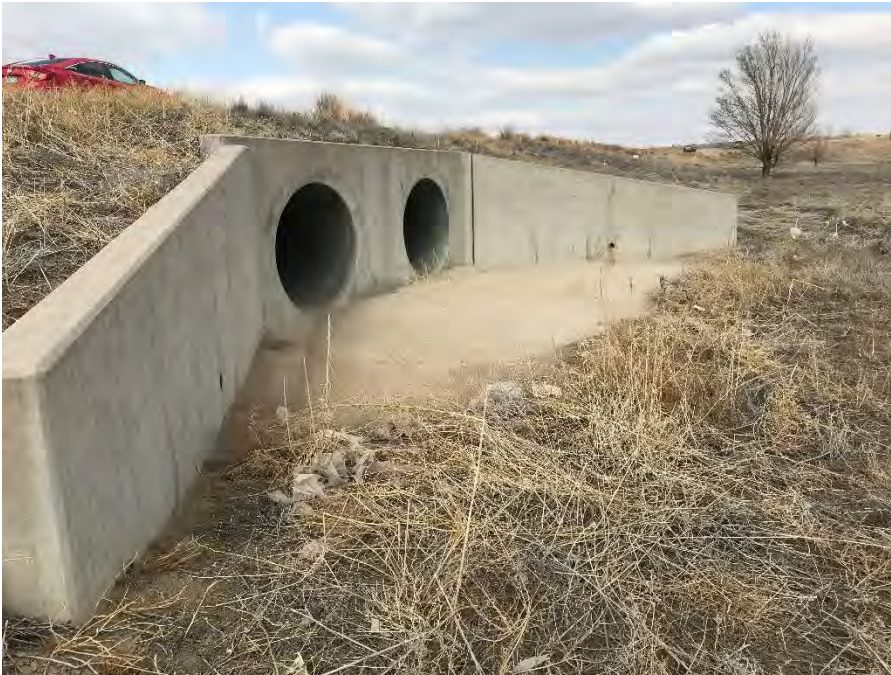
Photo 1: Standing at the northern side of the Property, looking north, towards the culvert crossing.
