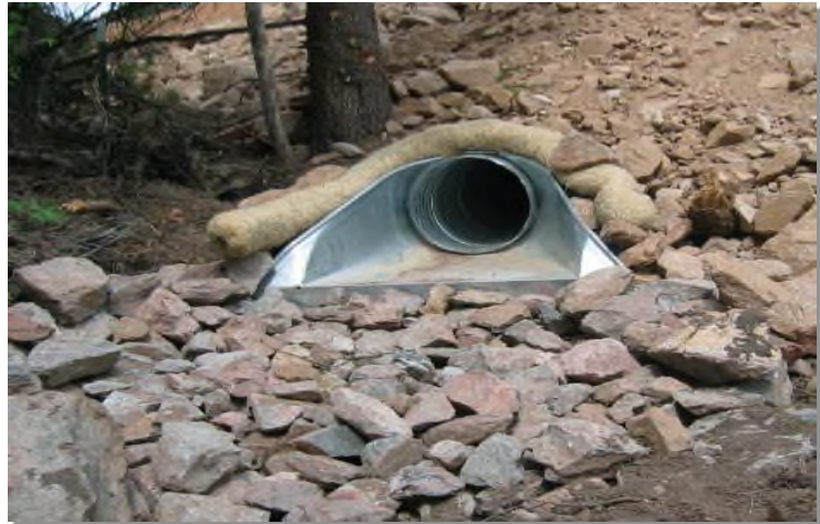
Photograph TOP-1. Riprap outlet protection.
