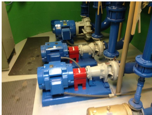
Figure 7: PBHMD Booster Pumps
