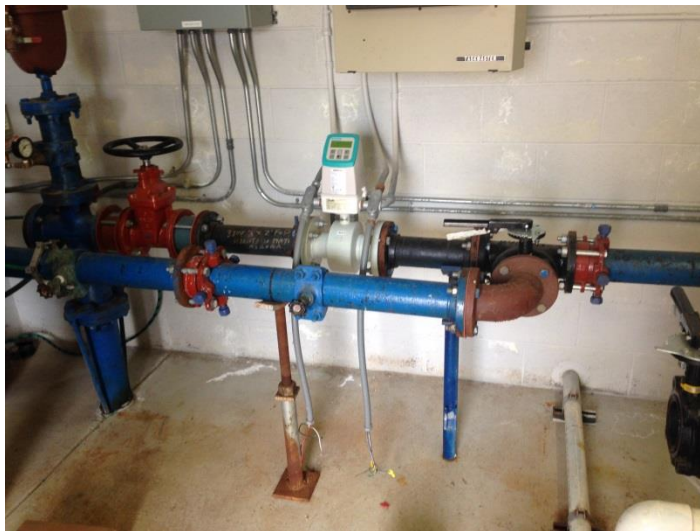
Figure 5: Piping inside Pump House 6
