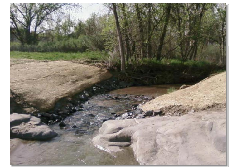
Photograph SS-1. Streambank stabilization using geotextiles following installation of a permanent in-stream grade control structure.
