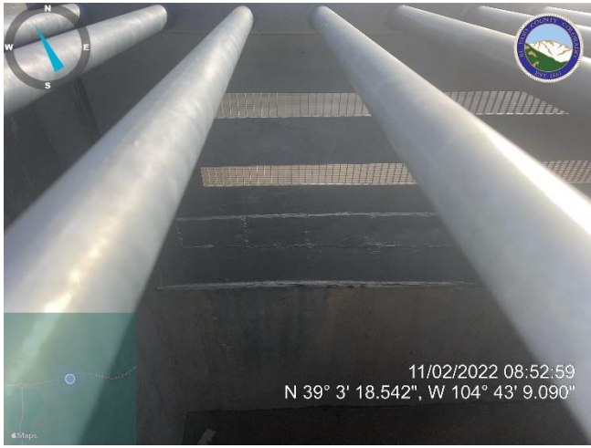
Photo 3: Irrigation Reservoir Embankment (JD Pond 13) 8'x4' SWQ Outlet Box with flow control plate welded shut.
