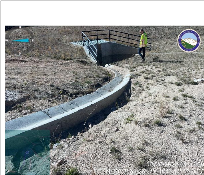
Photo 1: Raise pond bottom to meet top of trickle channel at Detention Facility 4
