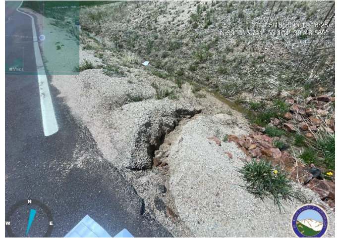
Photo 2: Fill erosion occurring along road shoulder of Sanctuary Pine Drive.
