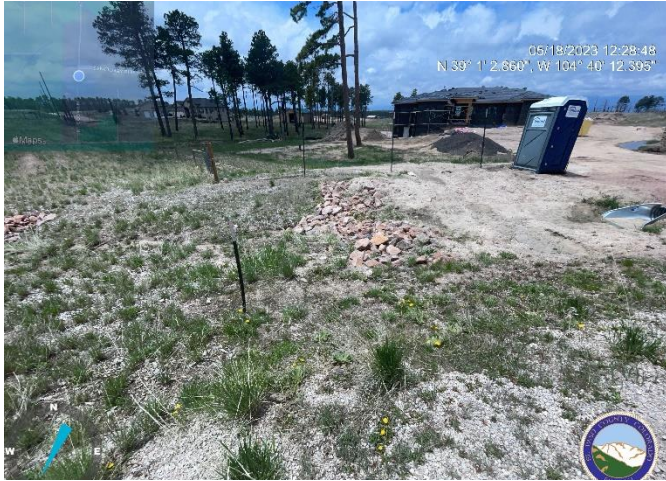
Photo 1: Sediment entering extended detention basin 1 at rock check dams at 12804 Ward Lane.
