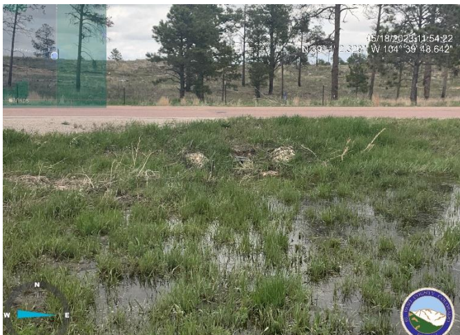
Photo 3: Remove rock socks from culvert under Vollmer Road; regrade so that no ponding occurs. All temporary control measures must be removed prior to FA.
