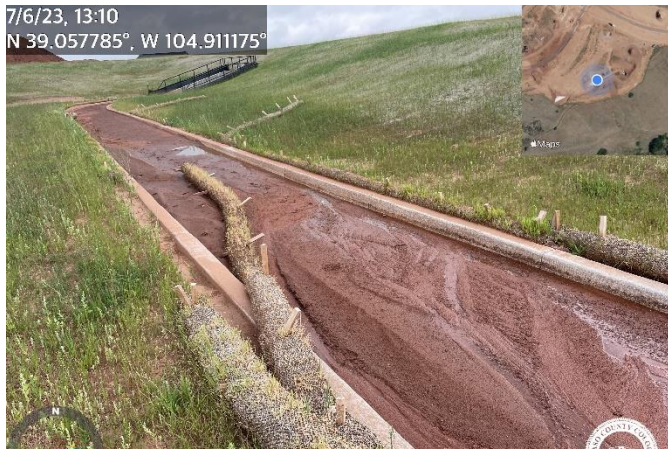
Photo 1: Remove sediment from trickle channel, forebay, and outlet structure of detention facility A.
