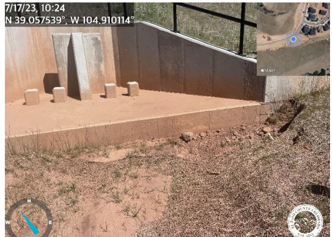
Photo 2: Backfill scouring along base of 30" RCP baffle structure on sheet 23 of 31.
