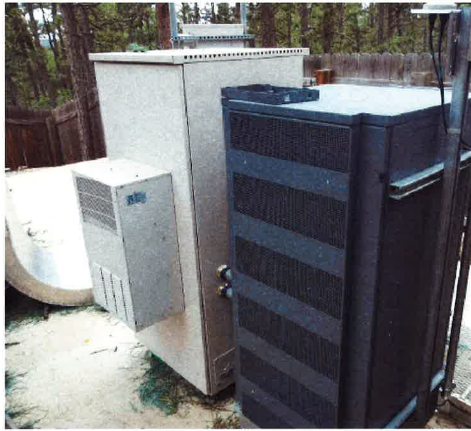
1 T-MOBILE EQUIPMENT PHOTOS A-1.1
