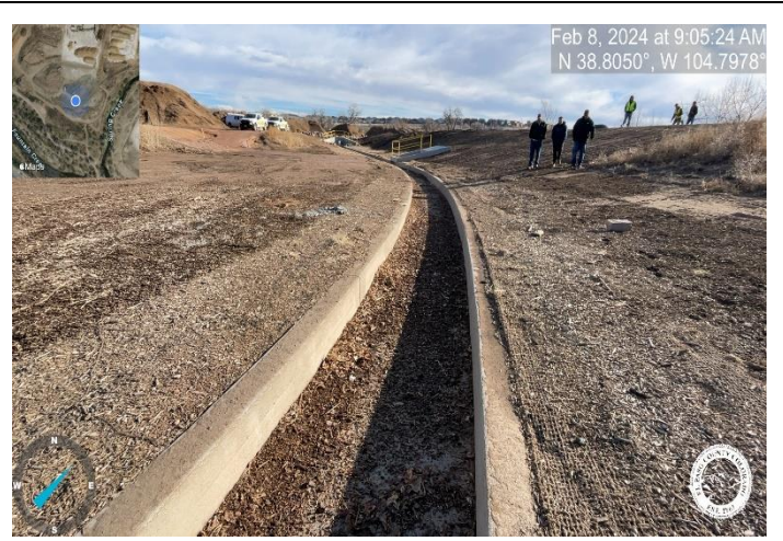
Photo 2: Clean out sediment and debris from the forebays, outlet structure and trickle channels.
