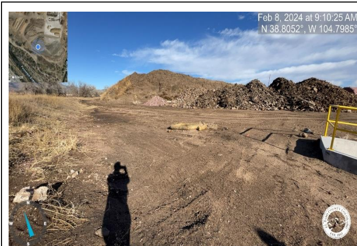
Photo 3: Flow currently bypasses inlet behind the west forebay. Regrade to promote flow into type D inlet.
