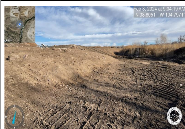
Photo 1: Pond: Grade the bottom of the Spillway to match slope shown on the Extended Detention Basin and GEC Plans. Reference sheet 3.
