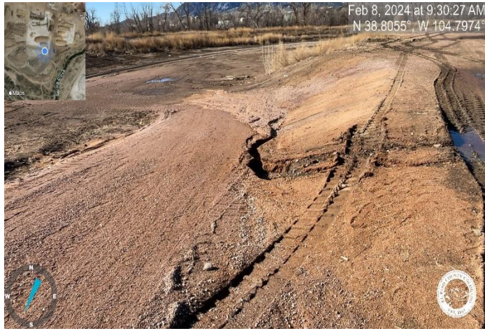
Photo 6: Repair rilling along maintenance access road. Rilling could worsen and will be required to be repaired at Final Acceptance.
