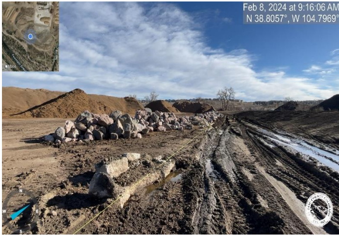
Photo 7: Complete installation of the 77 CY Riprap check (208'x10'x1' thick). Reference sheet 2 on the Extended Detention Basin and GEC Plans.
