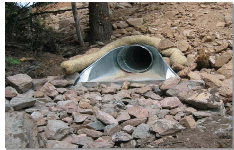
Photograph TOP-1. Riprap outlet protection.
