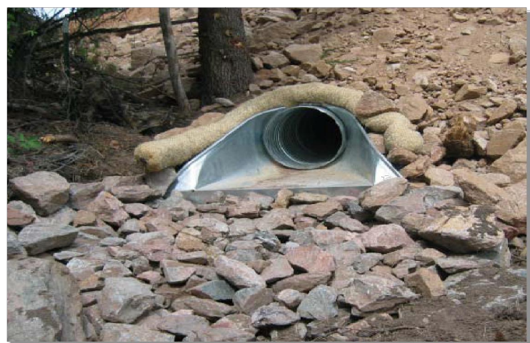
Photograph TOP-1. Riprap outlet protection.
