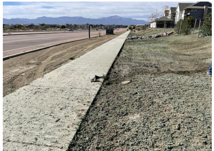
Photo 4: Bring grade up at south end of site to be flush with curb and sidewalk to prevent standing water in right-of-way.
