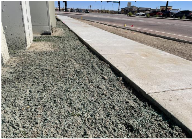
Photo 5: Bring grade up at south end of site to be flush with curb and sidewalk to prevent standing water in right-of-way.
